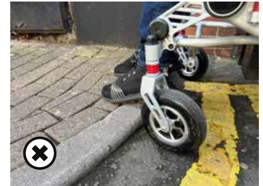
Lack of drop kerbs / level access
