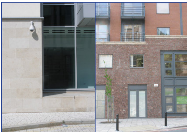
Contemporary interpretations of the traditional use of stone for cladding the lower storeys of buildings. A dense hard stone is advised, especially up to 600mm above the pavement surface, in order to resist the effects of impact, damage, splashback and salting and gritting of pavements or roads
