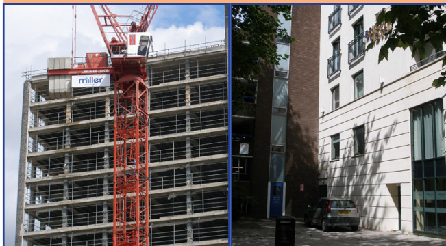
Left: new frontage being fitted around existing frame. Right: New hotel built onto the front of existing building.
