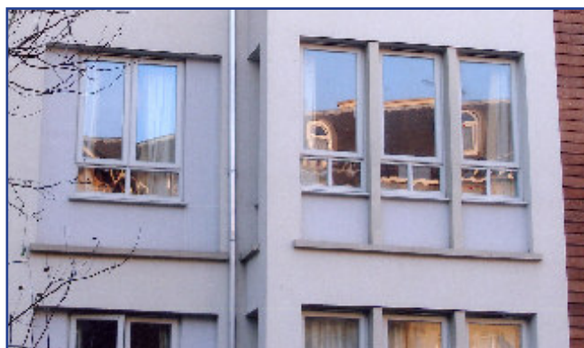
Well articulated and proportioned powder coated steel windows on a rendered elevation. Cedar boarding however is considered inappropriate in an urban location.
