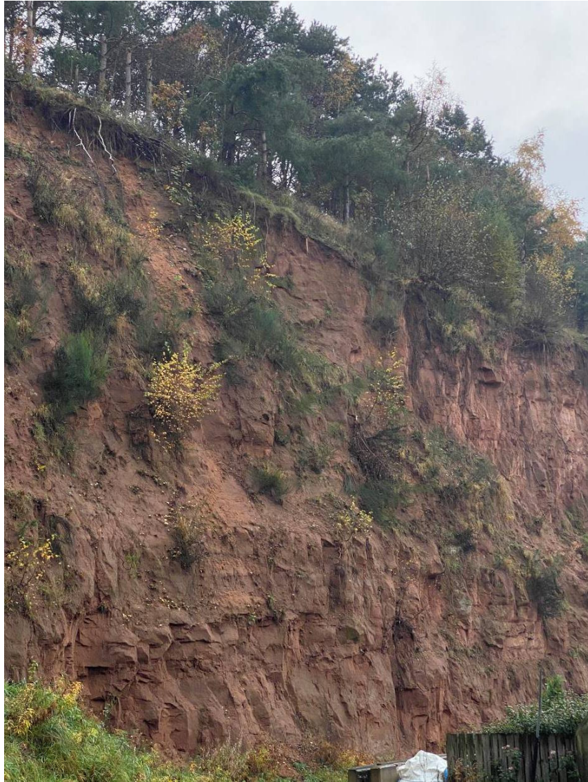
Photograph 4: Looking at the western flank. Evidence of overburden spalling from upper cliff face in Unit 8 as identified on 3 rd November 2020 (Image taken on 10/11/2020).
