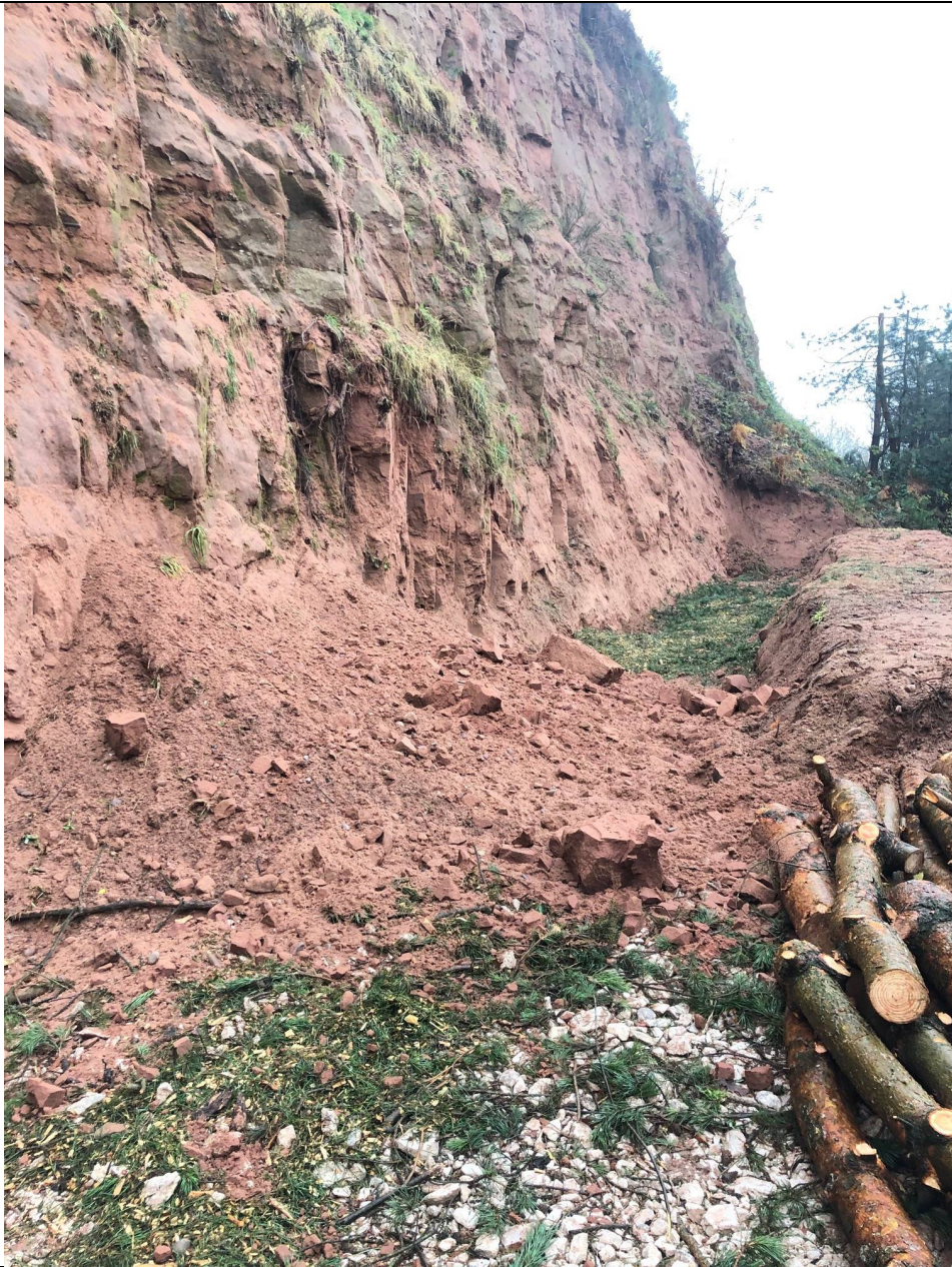
Photograph 3 : Debris at base of cliff face near extents of emergency work, to rear of No. 84 Stone Bank
