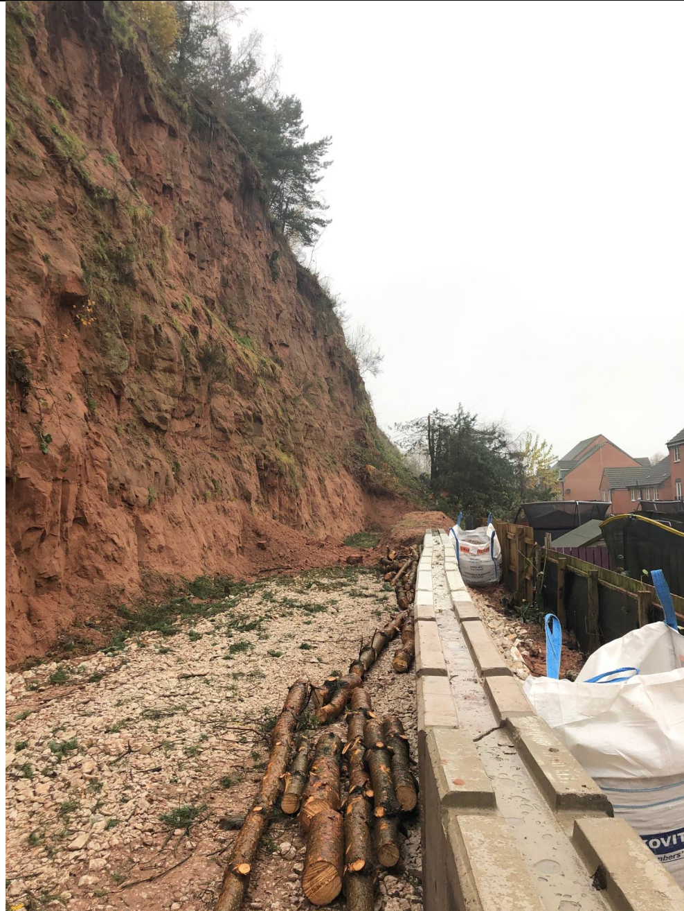
Photograph 2: Debris material contained within rock trap
